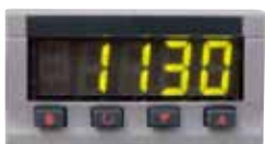
Over-temperature limit controller
