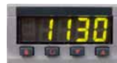
Over-temperature limit controller
