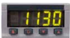
Over-temperature limit controller
