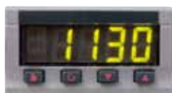
Over-temperature limit controller
